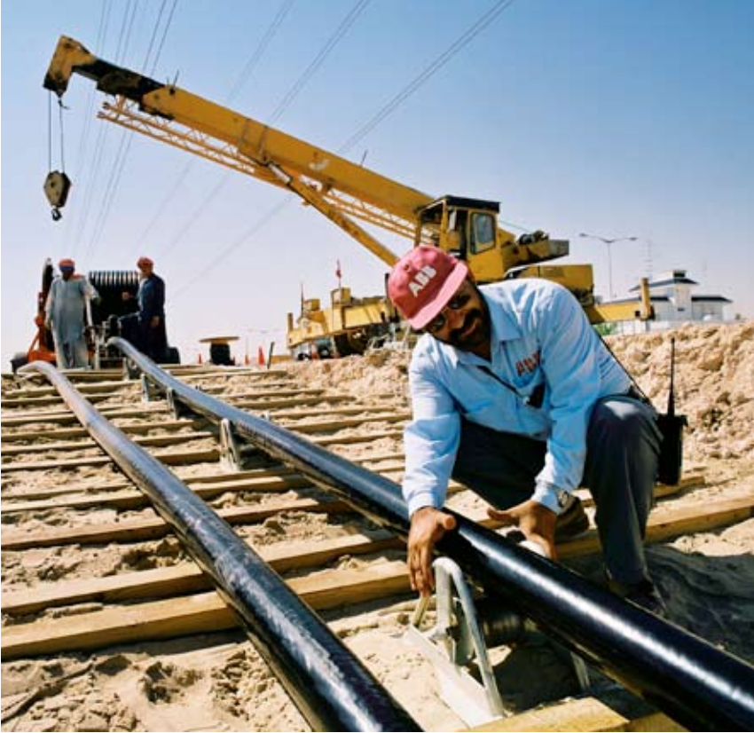
Laying underground high voltage cable from ABB, for reliable and invisible power transmission.
